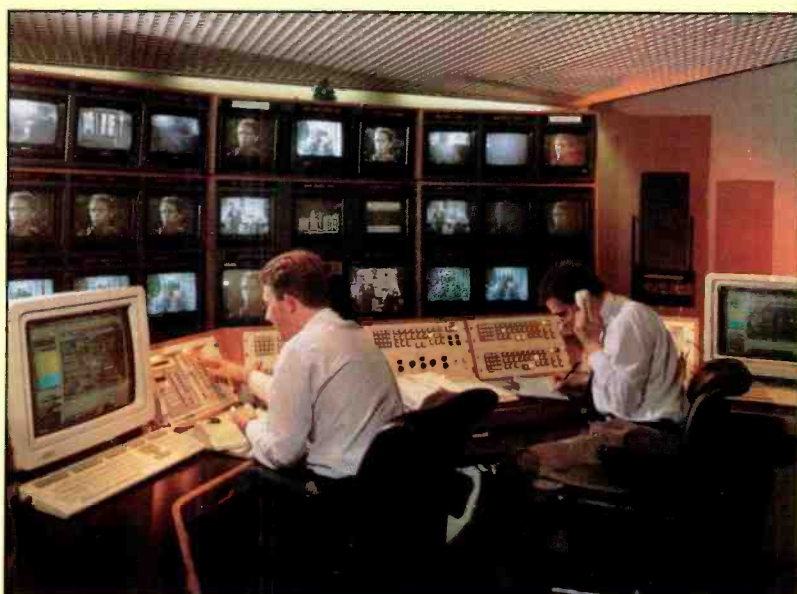
Regional Operations Centre (ROC) at Emley Moor in North Yorkshire controls commercial TV transmissions for the midlands and north of England.
