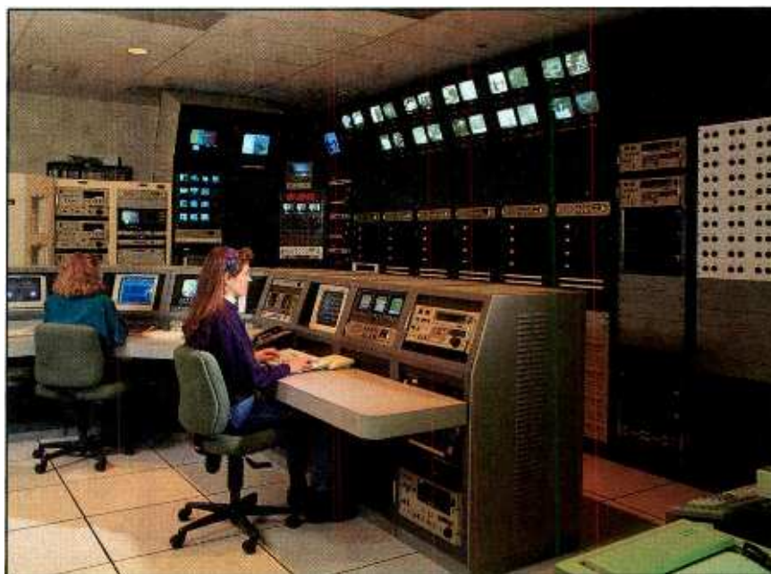
StarNet control room in West Chester, PA, monitors and retransmits all ad-supported cable network cue tones and deploys an MPEG digital uplink to send commercials to affiliates for storage and playback.
